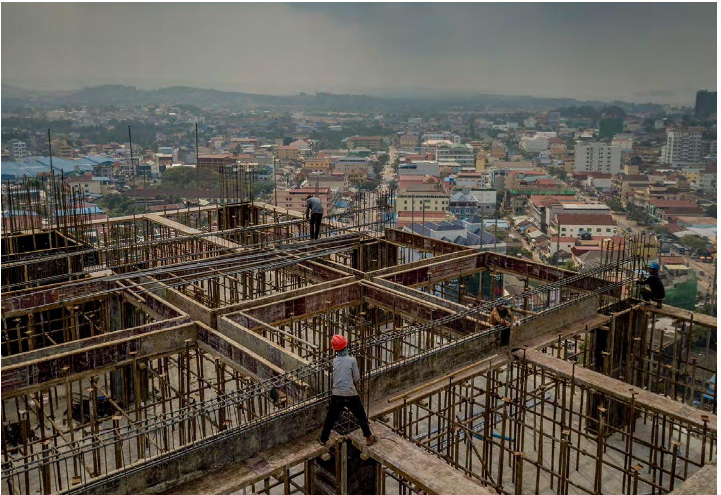
Construction workers on a new Chinese-financed casino, condo, and hotel development on the seafront in Sihanoukville, Cambodia, on February 17, 2018. During the COVID-19 pandemic, developments like this were converted into militarized scam compounds. (Photo by Adam Dean/New York Times)
