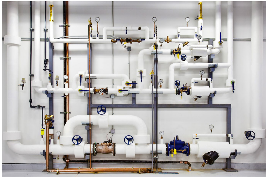
We keep pipes like these at our Douglas County, Georgia, data center ready with highly pressurized water in case of a fire.
