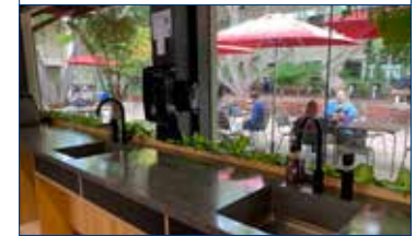
Kitchens provide boiling & chilled filtered water
