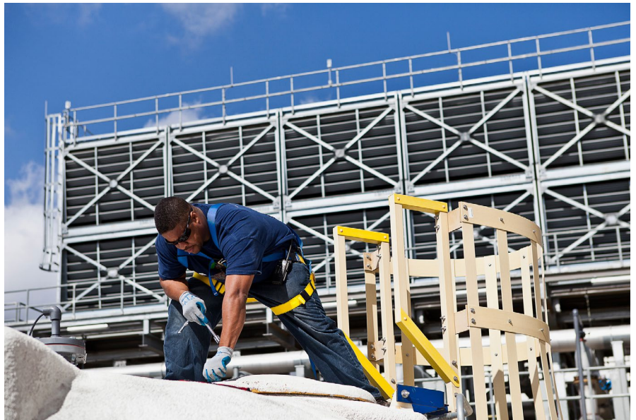
An employee works atop a storage tank at Google's data center in Douglas County, Georgia.
