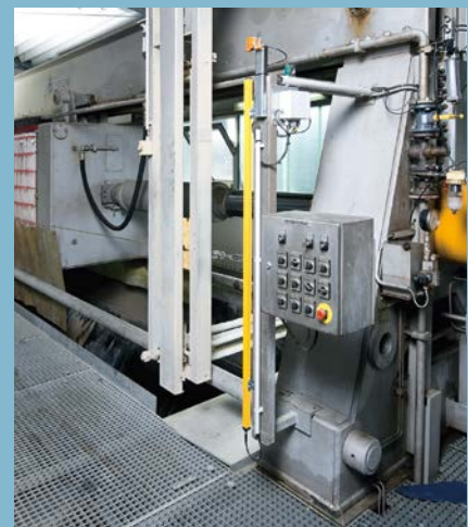
Safety monitoring of a chamber filter press.
