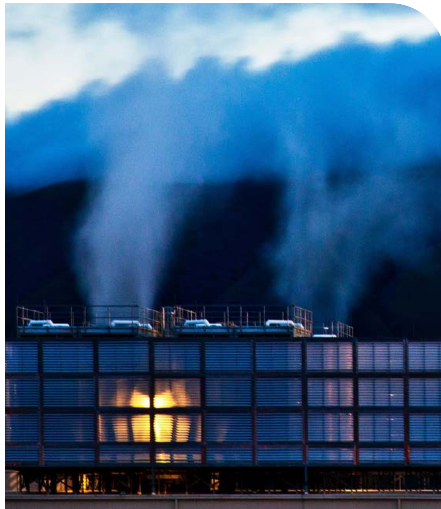
Steam rises above the cooling towers at our data center in The Dalles, Oregon.
