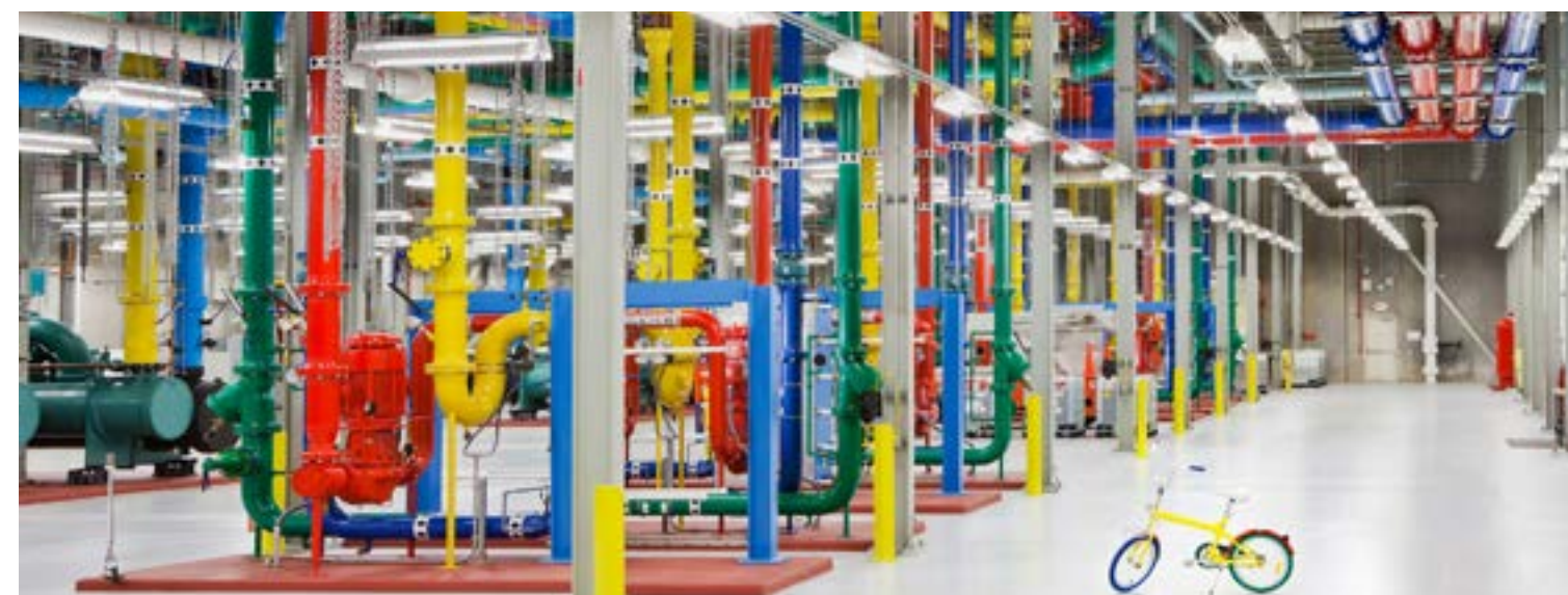
These colorful pipes in our Douglas County, Georgia data center send and receive water for cooling our facility.
