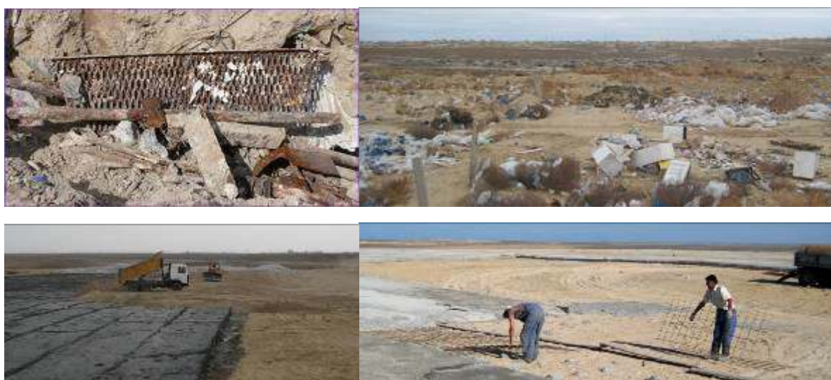
Figure 7. General view on the Koshkar-Ata uranium residue tailings bear Aktau city (western Kazakhstan) with still recently allocated radioactive waste storage facilities derived from the Caspian Hydrometallurgical Plant before and after partial remediation done in 2009.
