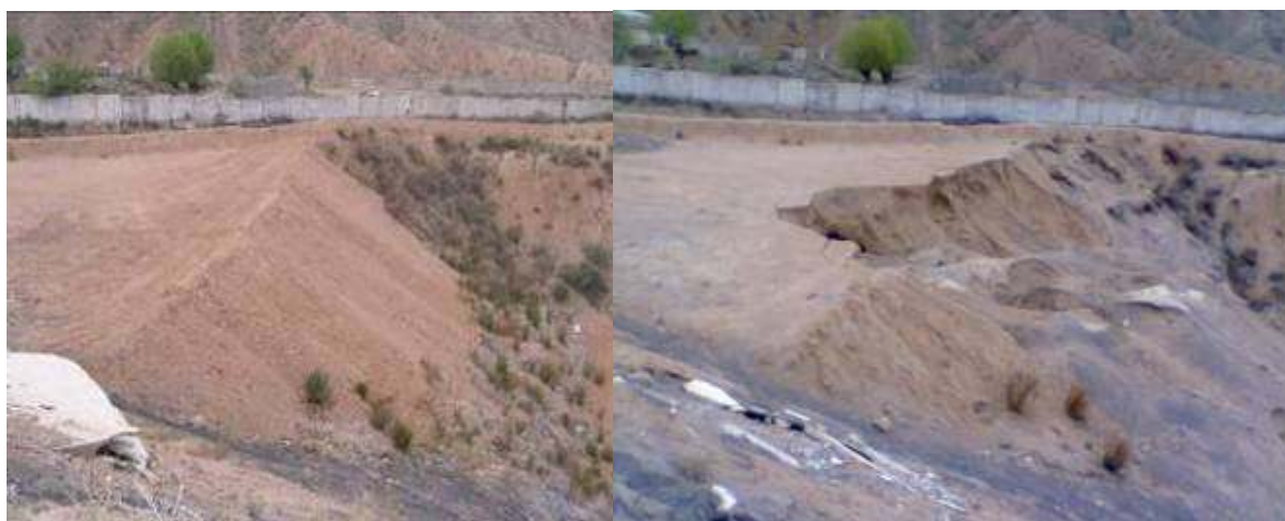
Figure. 13. The cover of the ash tailings (left photo) at the Kadji-Say facility were built in 2005 (the photo taken in June 2006). The same cover damaged by erosion, (see right photo, in April 2007), [15] (RER9086 Final Report in draft).
